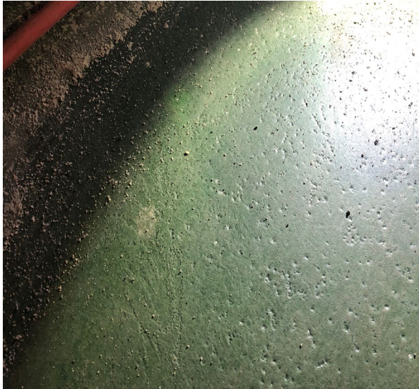
Figure 1 - Localized Corrosion Prior to Application of Steel-Filled Epoxy Putty
