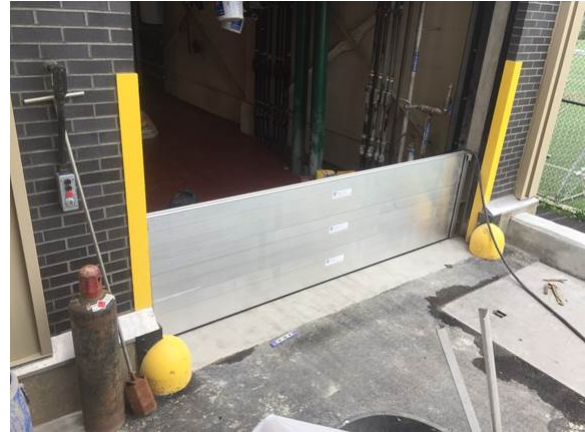
Figure 4 - Headworks Flood Barrier
