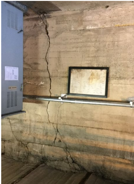
Figure 2: Bastion South Wall Crack
