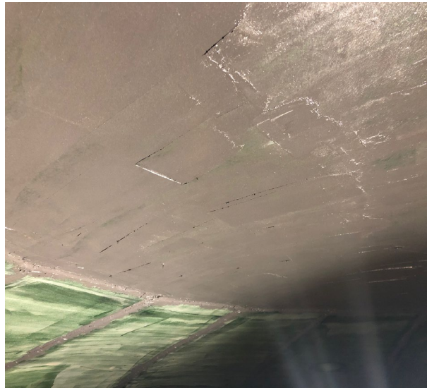
Figure 2 – Localized Corrosion after Application of Steel-Filled Epoxy Putty
